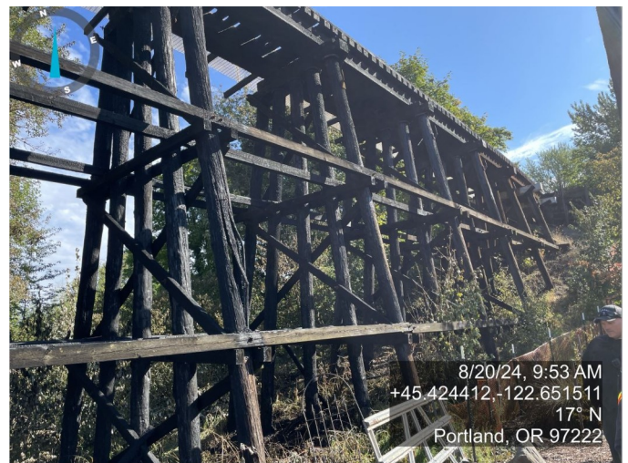
Charred components of structure
