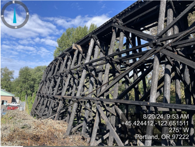
more photos of fire damage
