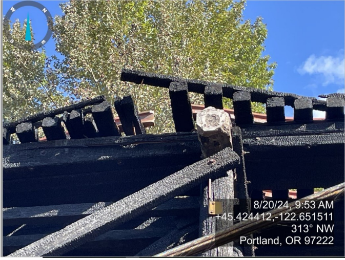
View of top and burned ties and broken rail
